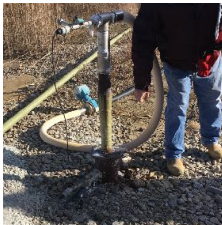
Wellhead of a solution-mined cavern producing industrial salt in Seville, OH
